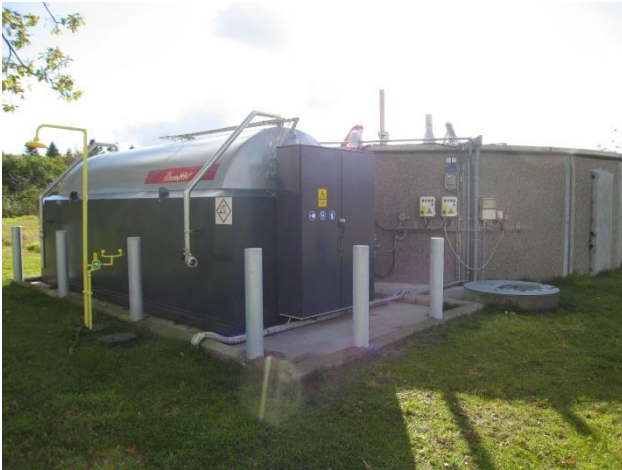
Figure 1. The “JH Forsuring NH4+” acidification system at location A.
