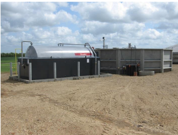
Figure 2. The “JH Forsuring NH4+” acidification system at location B.
